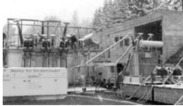
Figure 8: Off-line test set-up for PD-diagnosis on a 220/65-kV transformer using a 350 kVA diesel generator unit (left hand) and a step up transformer 0.4/65 kV (right hand). Transformer under test with torus electrodes at the HV-bushings to avoid corona discharges, and measuring vehicle (background).
